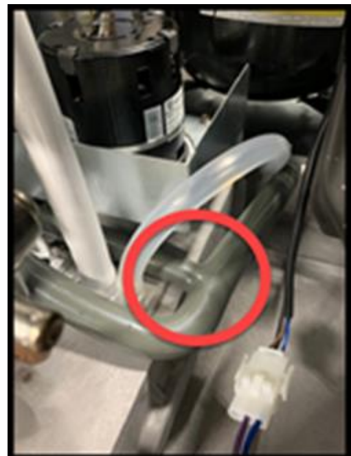
Figure 3: Intersection between drip tray and purge valve tubing
